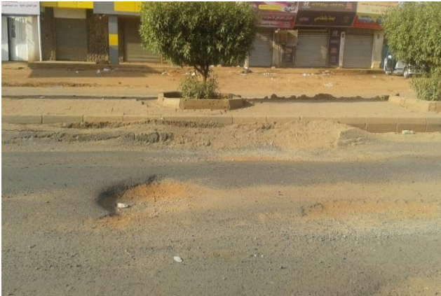
Plate 7. Sever failure of edgesand potholes.
