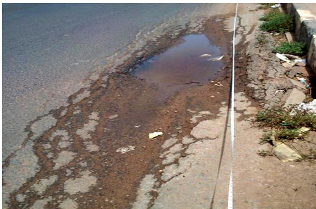
Plate 3. Severe pavement distresses of cracking, potholes and failure of edges.
