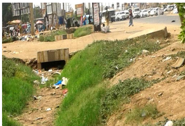
Plate 2. The side drain and the culverts were blocked with silt and sand accumulation, debris and vegetation.
