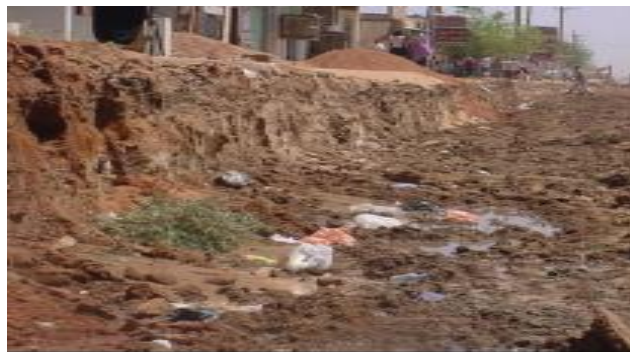
Plate 4. Accumulation of subsurface water on the sub grade of expansive soil.
